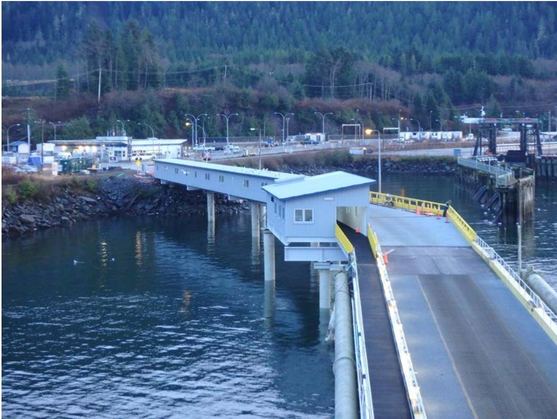
The new vehicle access ramp, covered customer walkway and waiting room at BC Ferries' Prince Rupert terminal.
